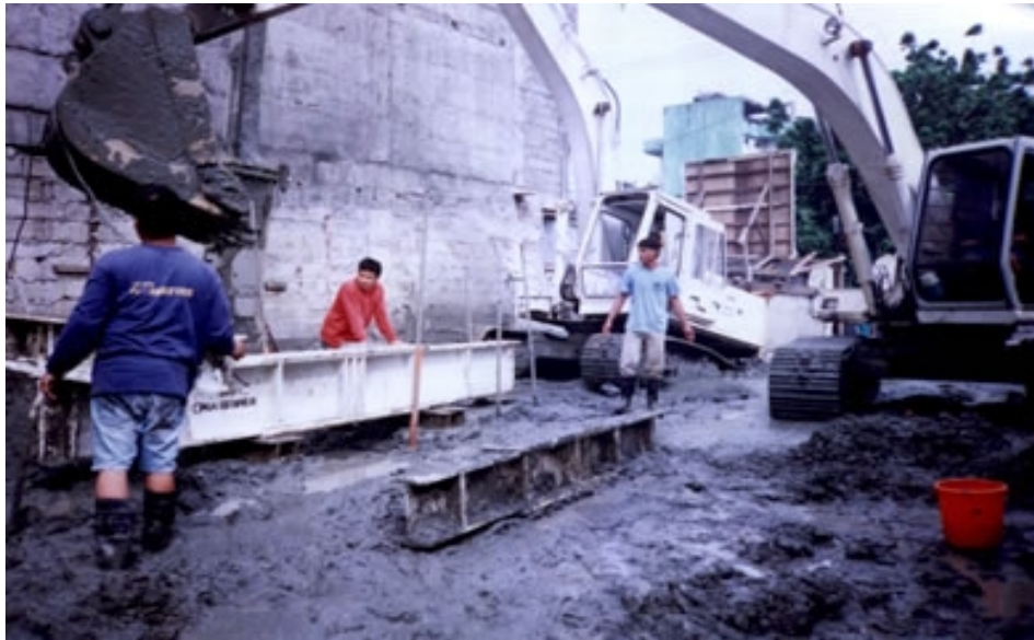
PGA Geopier crew setting up Modulus Load Test Frame for Stalder Project Result of Modulus Load Test
