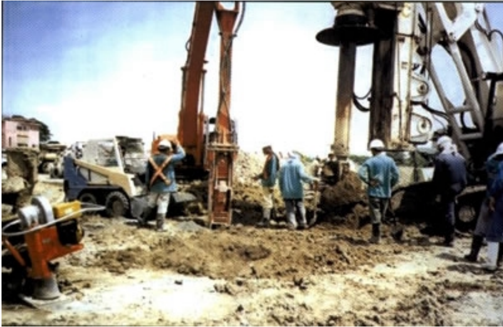
PGA Geopier crew on the job at S & R Ortigas, Pasig City
