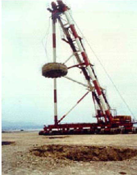
Figure 4.2.2.1 Mammoth DC Equipment
