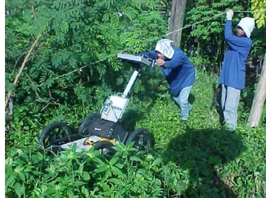
Fig. The GPR equipment being used scanning for Buried Pipes and aqueducts.
